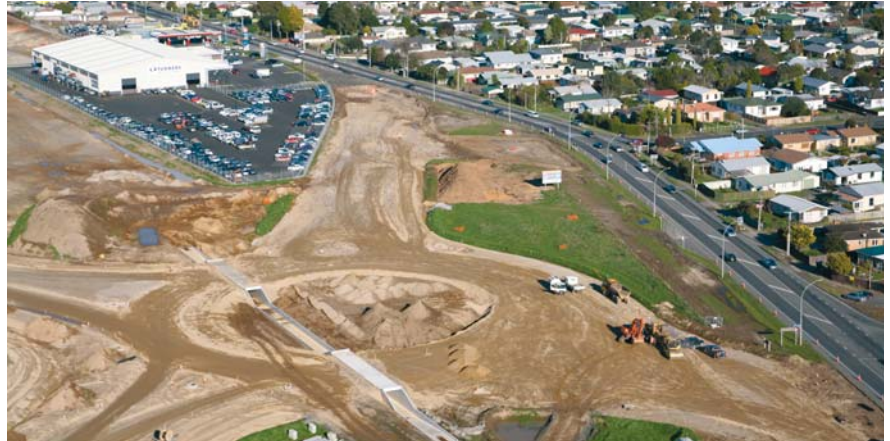
The Rotokauri roundabout takes shape beside Avalon Drive. The Avalon Drive Bypass begins at the bottom right-hand side of the picture and runs behind Turners Car Auctions (top left). Crawford Street connects with the roundabout at the bottom left-hand corner. Also visible are the pedestrian/cyclist underpasses, which will enable safe and easy crossing of the roundabout.
