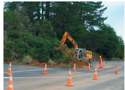
SH1 slip near Fryers Rd. The July storms compounded work to repair damage from storms earlier this year.
