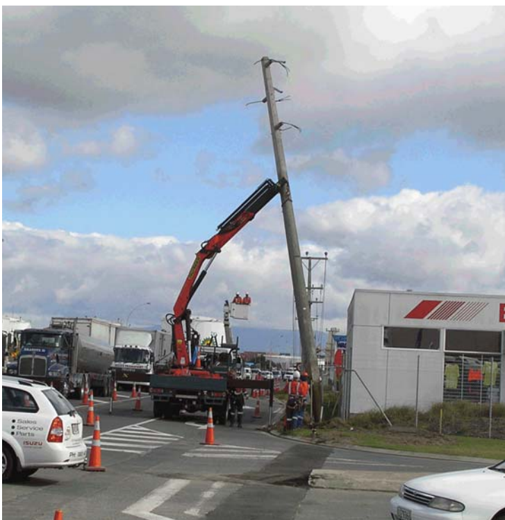
Left: North Power lifts out a power pole on Hewletts Rd. Power cables have been moved underground from Waimarie St intersection to Totara St.
